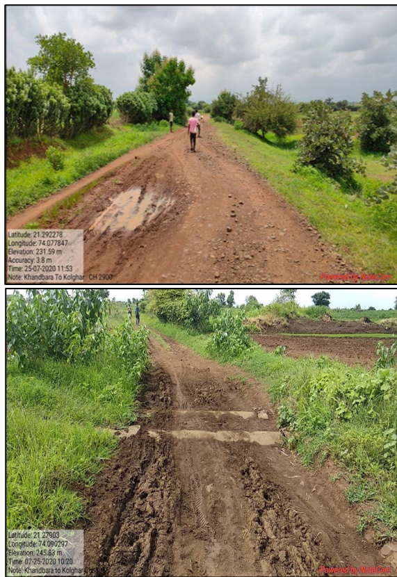
Fig. 1. Present condition of road
